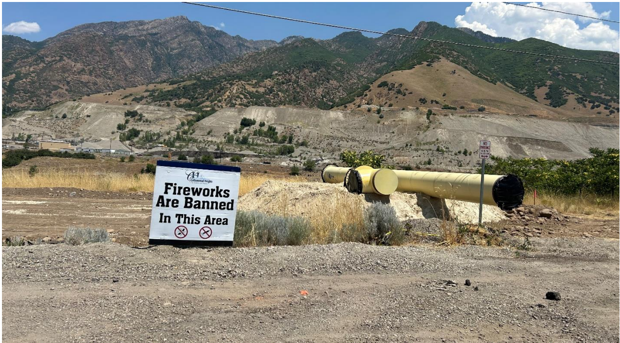
July 17: Grubbing, potholing, and pipe staging is beginning at Fort Union Blvd and Nutree Dr.
