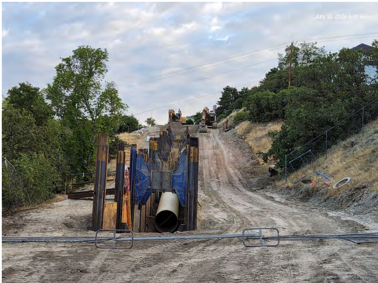
SLAR installation coming south / downhill from Deer Creek Road toward Danish Road.
