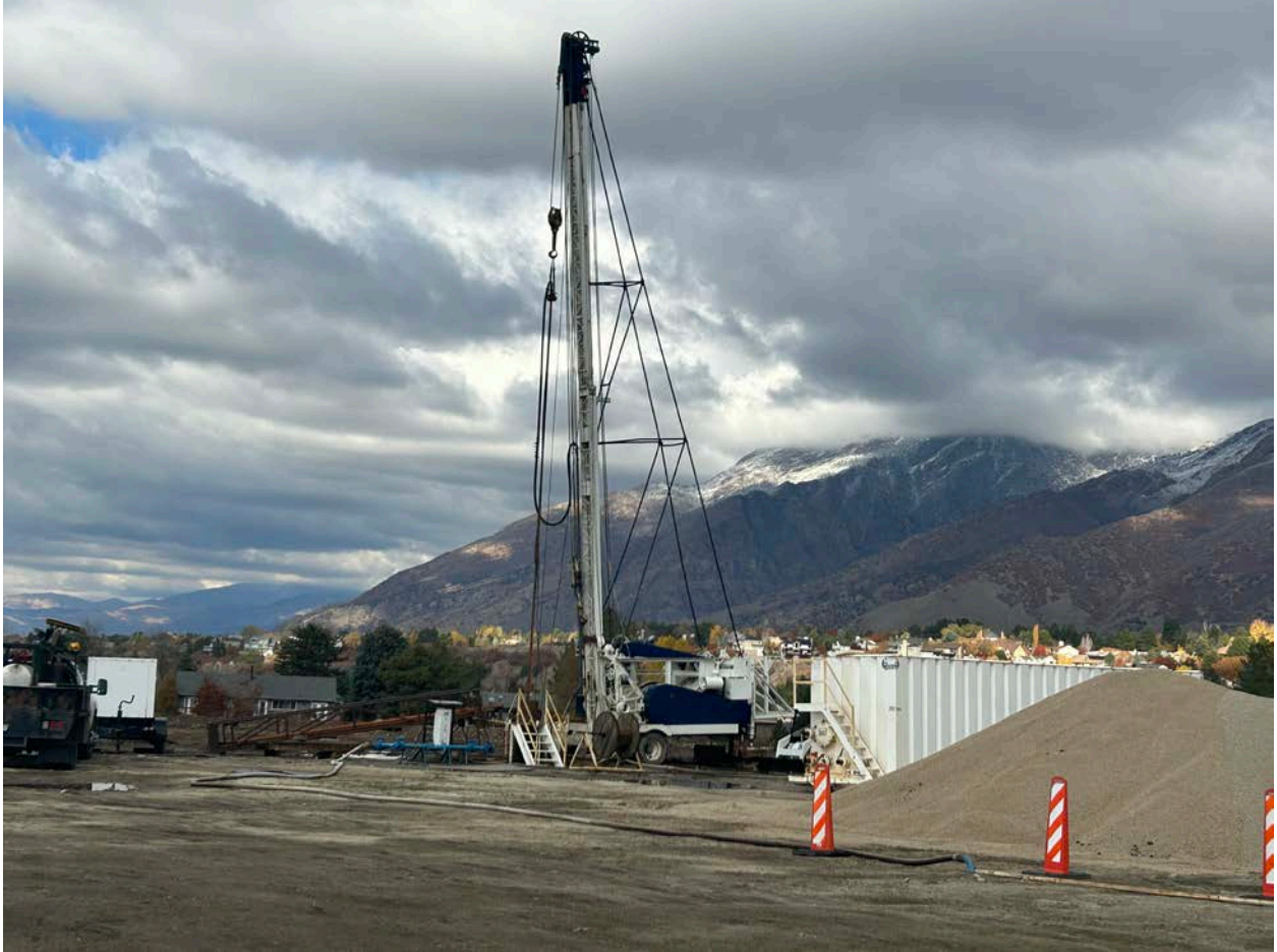
November 8: The ASR Well developing equipment is installed and swabbing the well. Swabbing is a process to kick-start the well by freeing up materials that are caught in the production zone.
